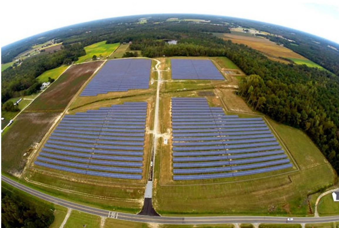
6.5MW system – S-Power, Selma, North Carolina
