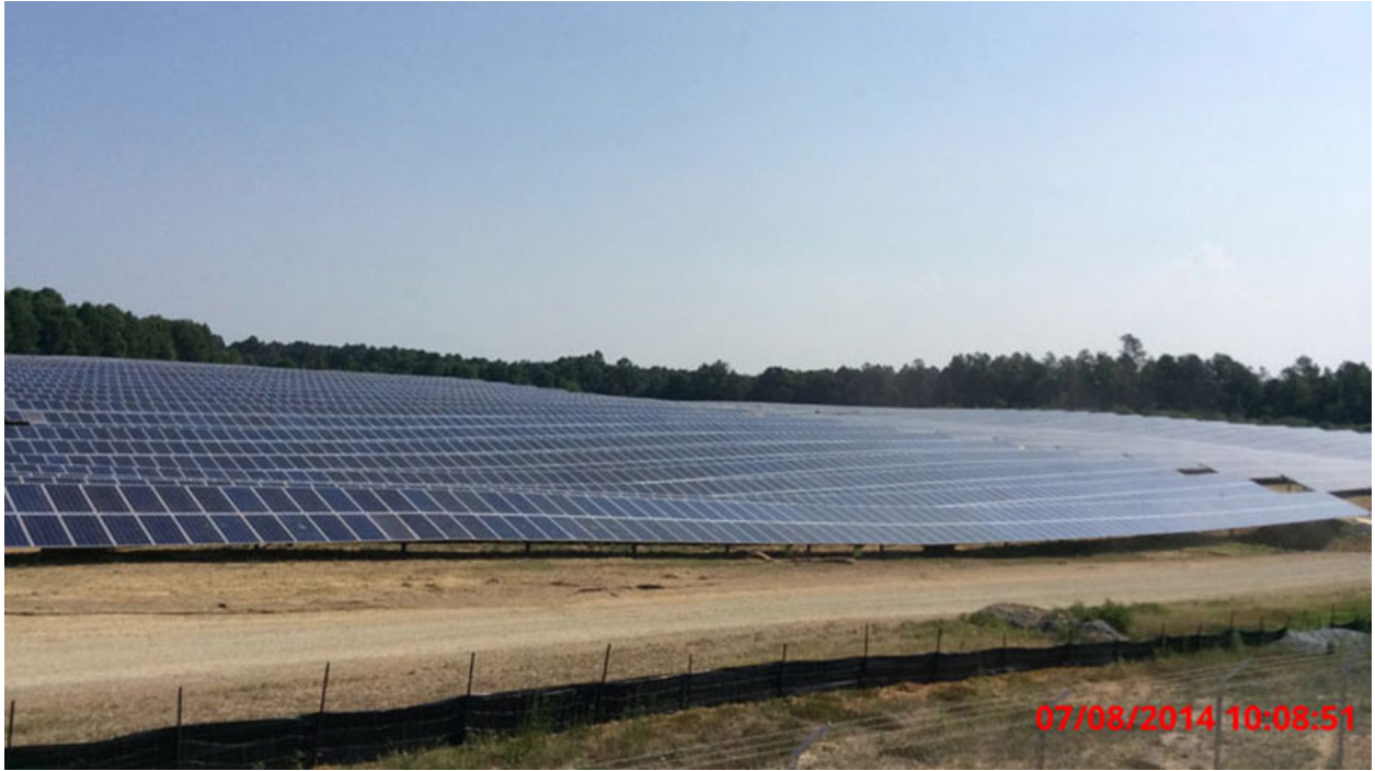
6.7 MW system – S-Power, Biscoe, North Carolina
