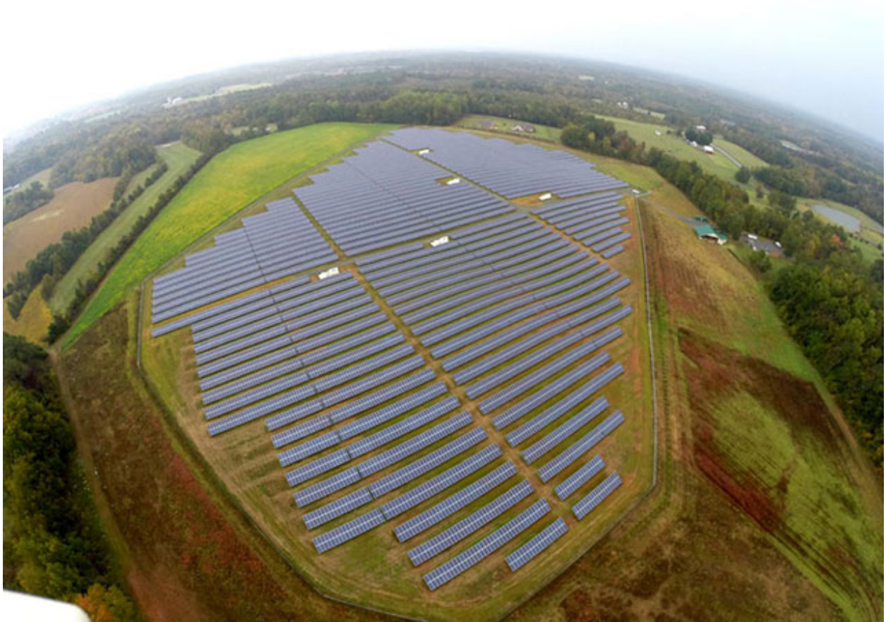
6.5MW system – S-Power, East Liberty, North Carolina
