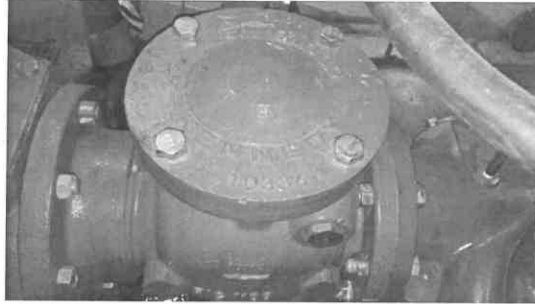
Figure 3.2: Insertion Check valve at Homestead Lift Station
