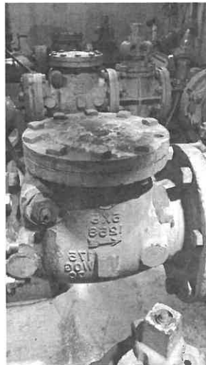
Figure 3.1: Insertion Check valve at Prospect Lift Station
