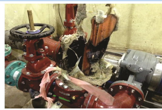
Pump failed due to clogging
