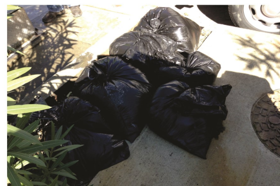
Five bags of wipes and debris from pump station cleaning
