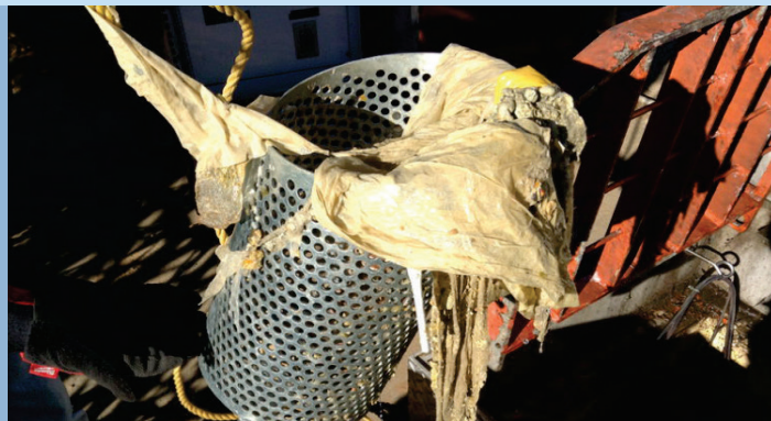
Wipes and Debris trapped in Pumps
