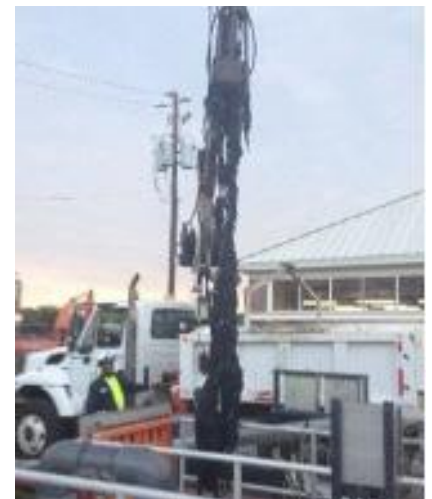
DC Water spent $100,000 repairing the Upper Anacostia Pumping Station after it was clogged with wipes.
