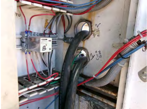
Pump Cable Entries
