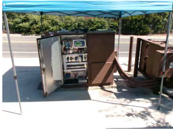
PLC and Utility UG Pull Section
