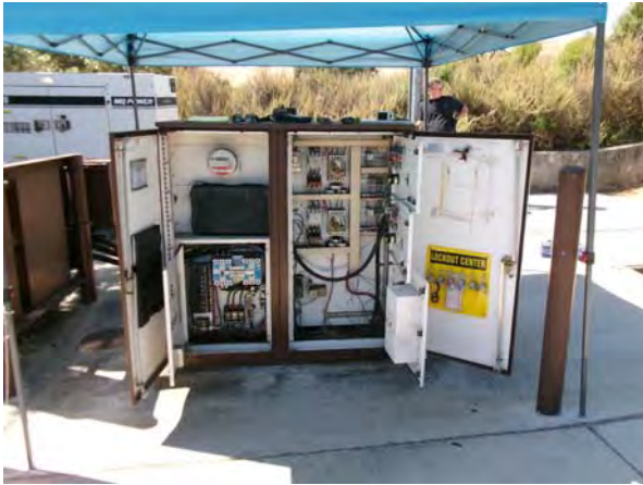
Power Distribution and Motor Controls
