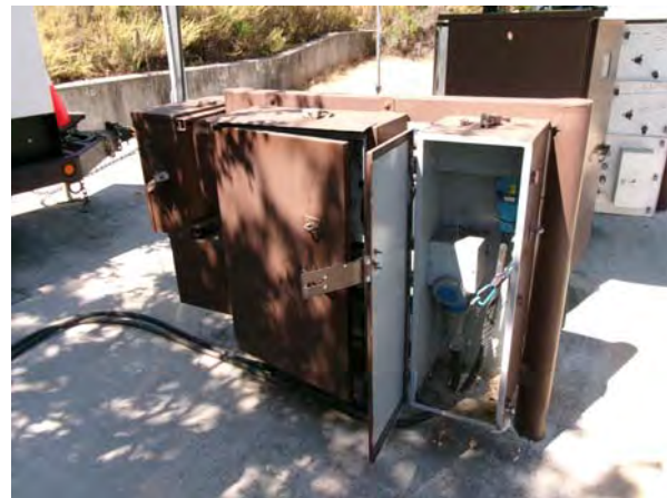
Generator Connection Panel and ATS
