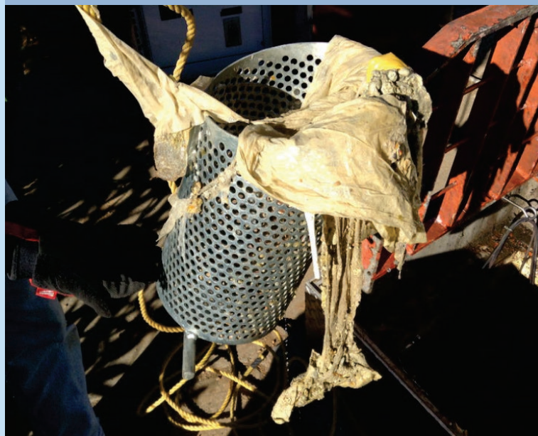
Wipes and Debris trapped in Pumps
