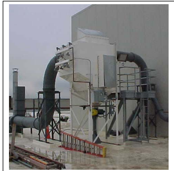
Roof top dust collector with explosion vents
