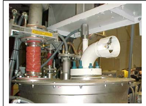
Sodium bi-carbonate active suppression on process vessel
