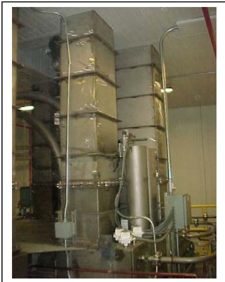
Stainless steel explosion vent ducts to carry products of deflagration to outside.
