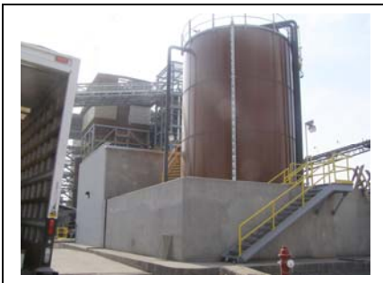
Above ground storage tank for No. 2 Fuel Oil
