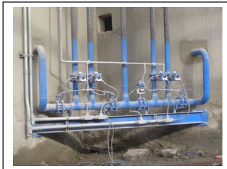
Compressed air piping manifold and control valves
