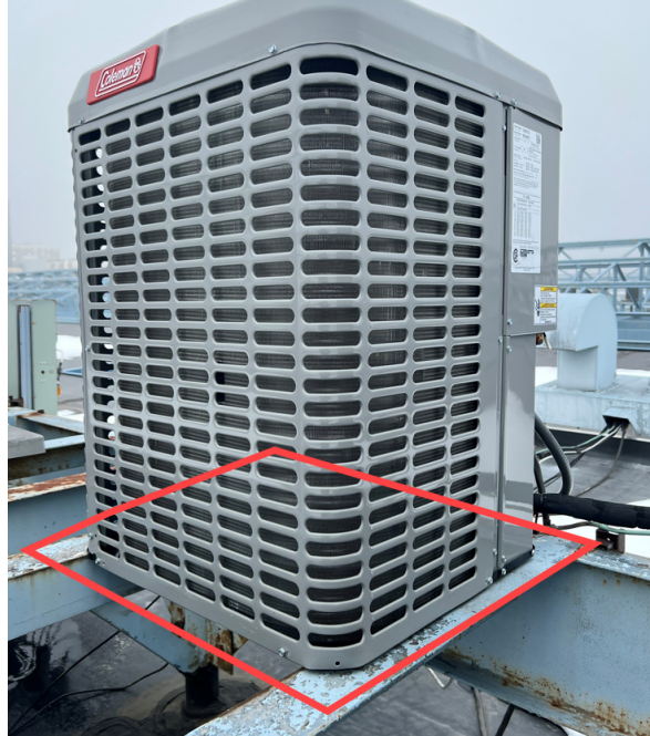
Figure 4. Example CU above Unit 434 rigidly bolted to dunnage
