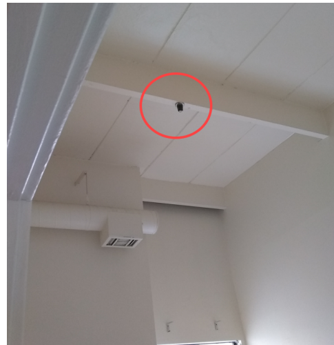
Figure 10. Node 3866 attached to Unit 403 ceiling structure
