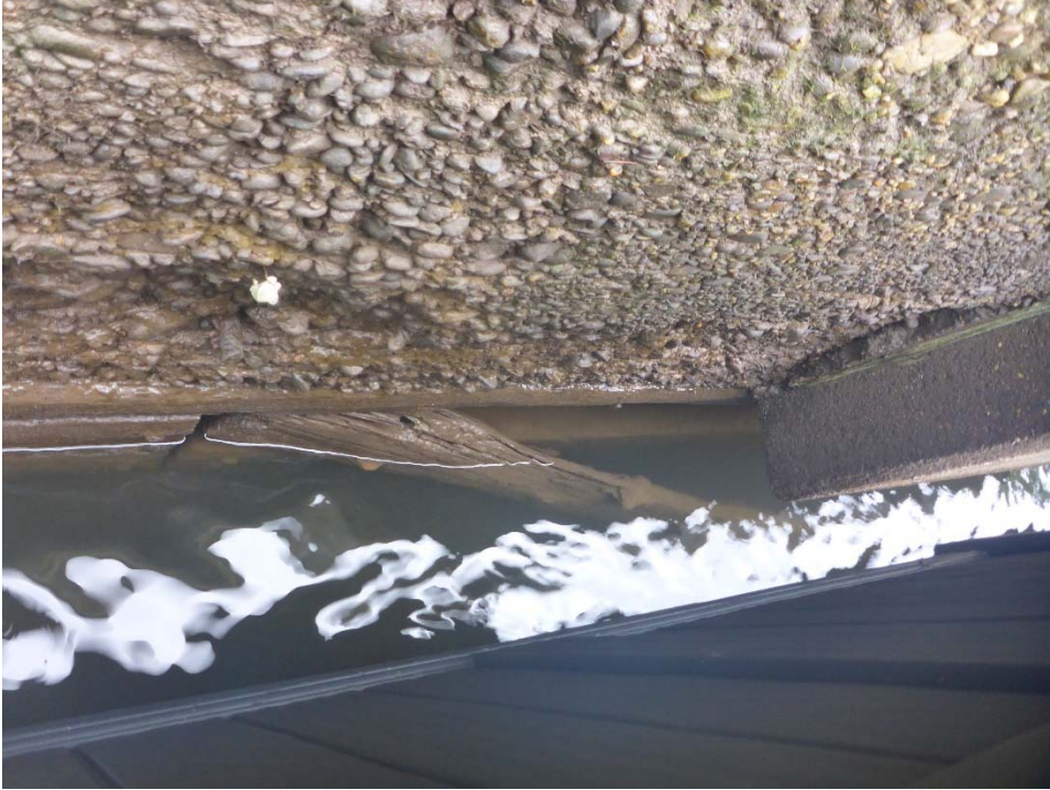
Photo 20: Typical broken skirt board on the north face.
