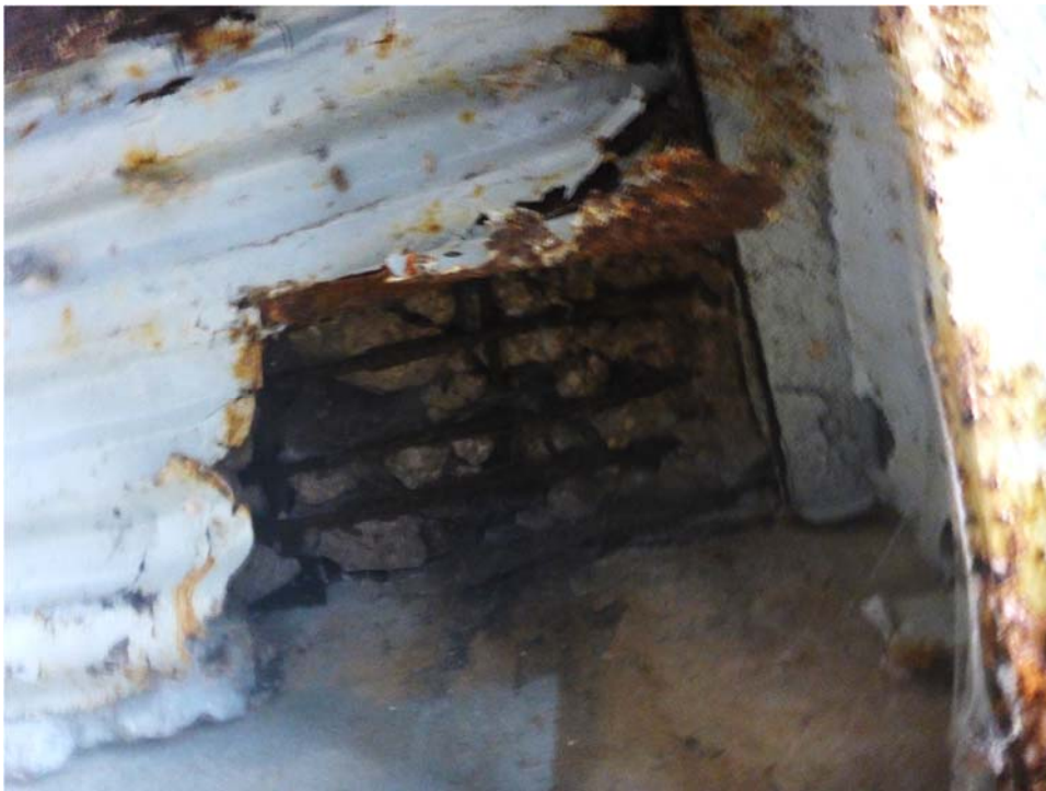
Photo 13: WD 1, northwest corner of bay 1, area of exposed and soft concrete with exposed reinforcing with up to 100% section loss.
