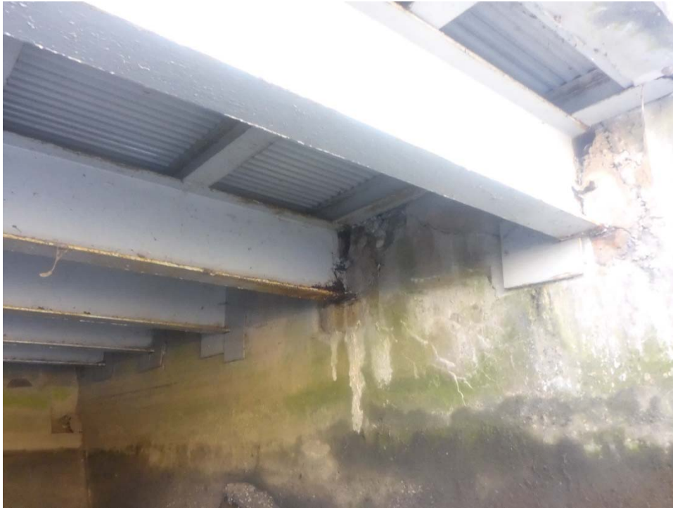
Photo 9: WD2, looking southwest. General layout of wharf drop 2. Note the SIP forms for the concrete deck and remnants of formwork that remain in place around the beam ends. Note that the stringers above the W18 beams are located in WD 2 only.
