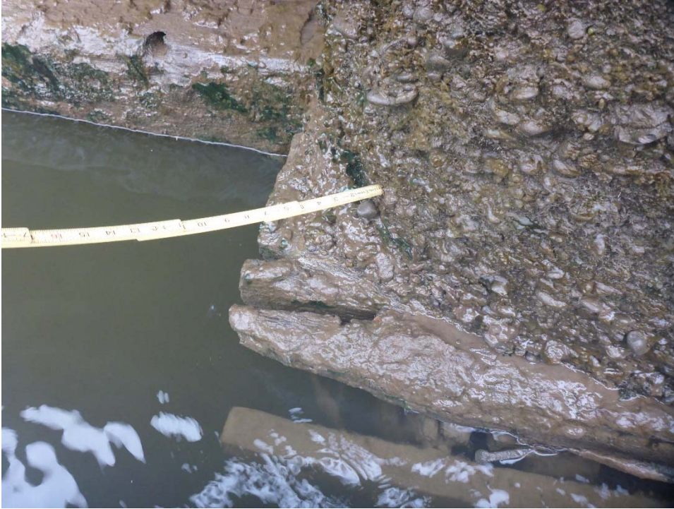
Photo 5: North face, spalling at the west corner of WD 3 measuring 48" H x 8" D with exposed and deteriorated deck. Similar deterioration was observed at each corner of the northern WDs.
