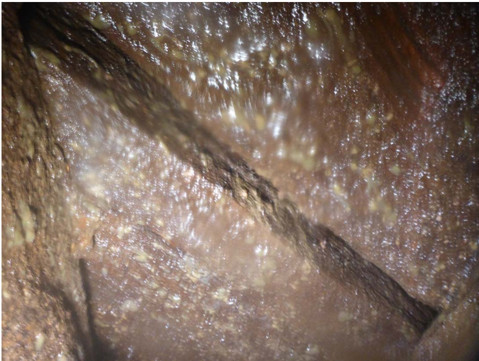
Photo 19: B/W bents 95S & 96S at Pile E. Gaps in timber deck up to 1" wide with no active loss of fill.
