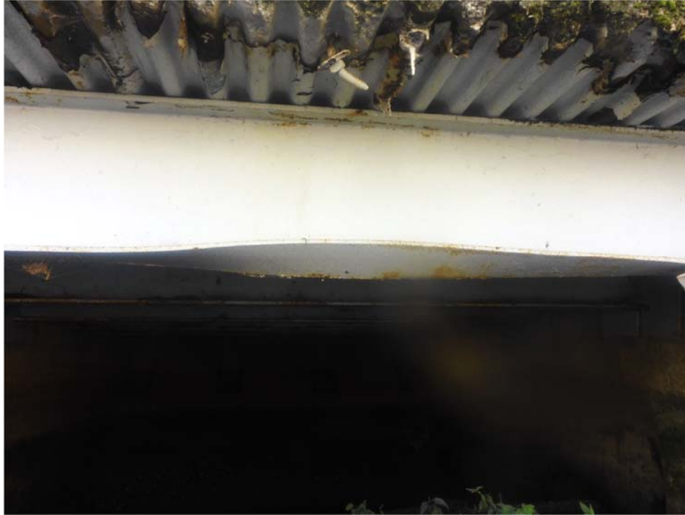
Photo 10: WD4, first beam from opening, looking south. Bottom flange was apparently struck previously. Note the deterioration in the SIP forms at the deck soffit.
