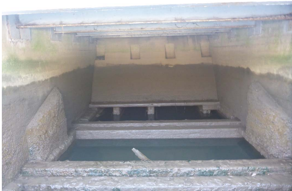
Photo 8: WD1, looking south. General layout of wharf drop. Note the steel beams spanning above and the sloped concrete back wall. Note the typical moderate abrasion that continues along the concrete walls.
