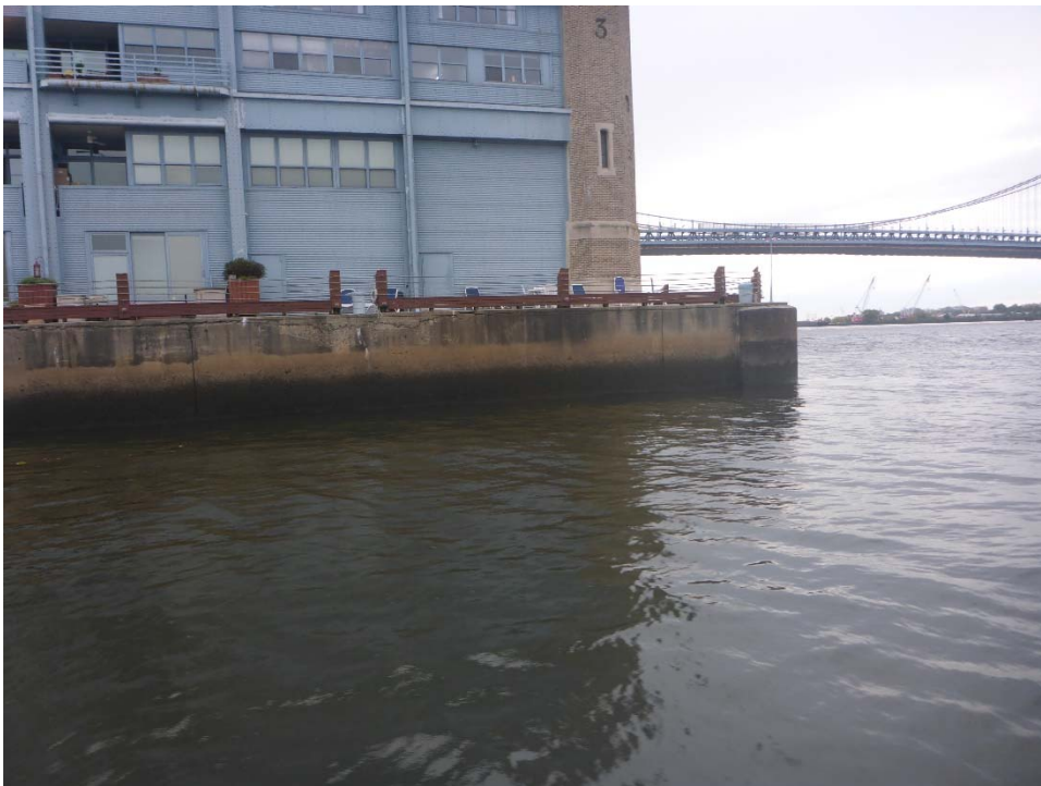
Photo 4: Typical section of south face of pier, east end, looking north. The seawall is in generally satisfactory condition. Note abrasion in lower 4' of the seawall.
