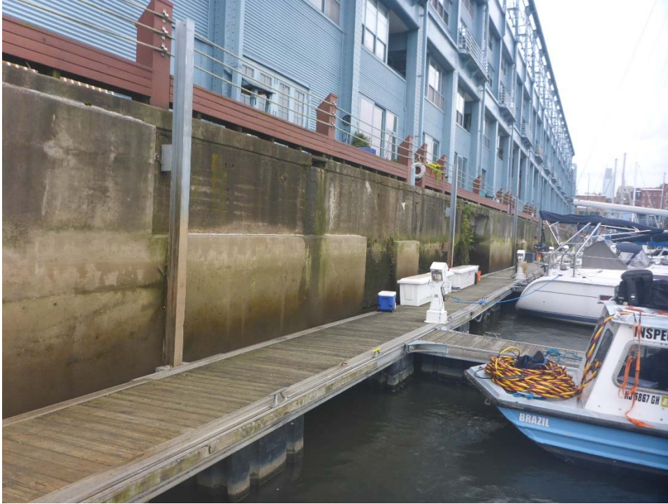
Photo 1: North face of pier, looking southwest towards WD 4. The seawall is in generally satisfactory condition, with hairline map cracking and light efflorescence throughout. Random areas of the seawall have been repaired.
