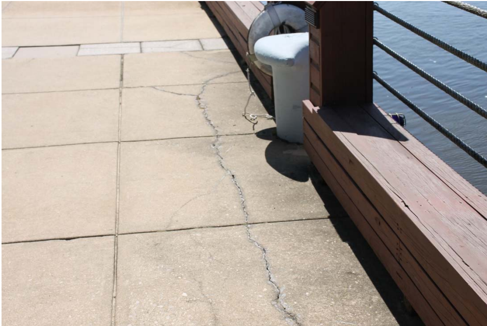
Photo21: South side of the pier, looking southeast. Typical cracking up to 1/8" W.
