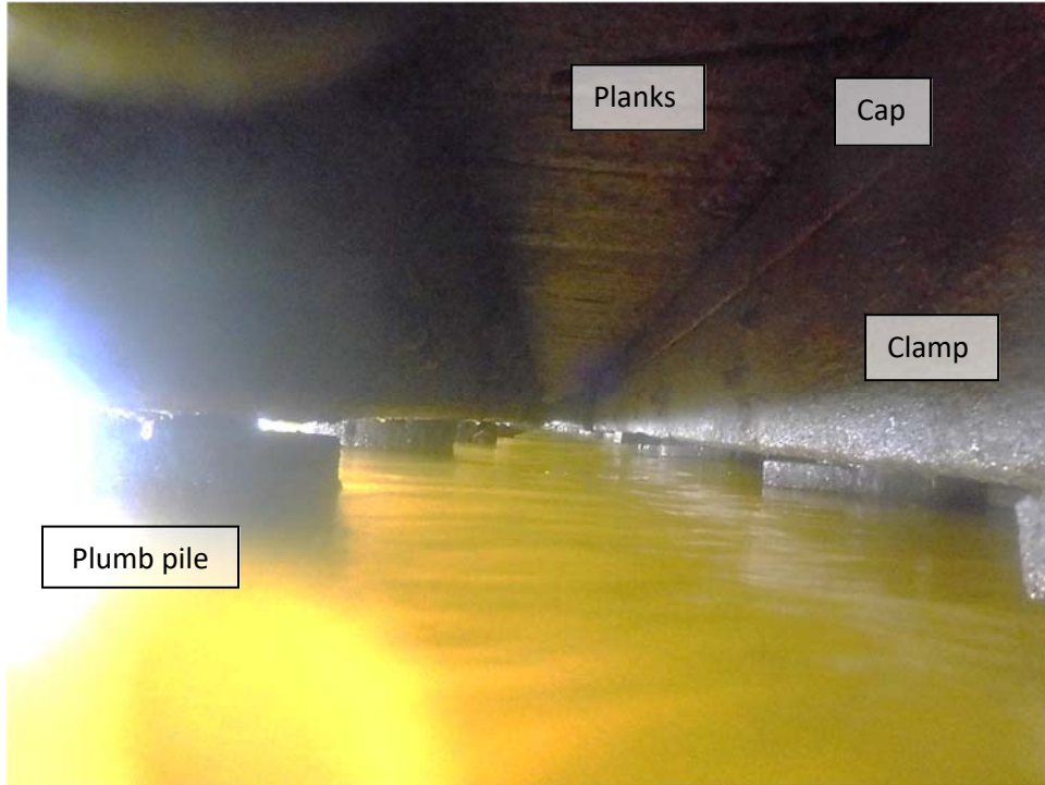
Photo 14: Bay between Bents 1 1/2', looking south. Typical layout of timber low deck elements.
