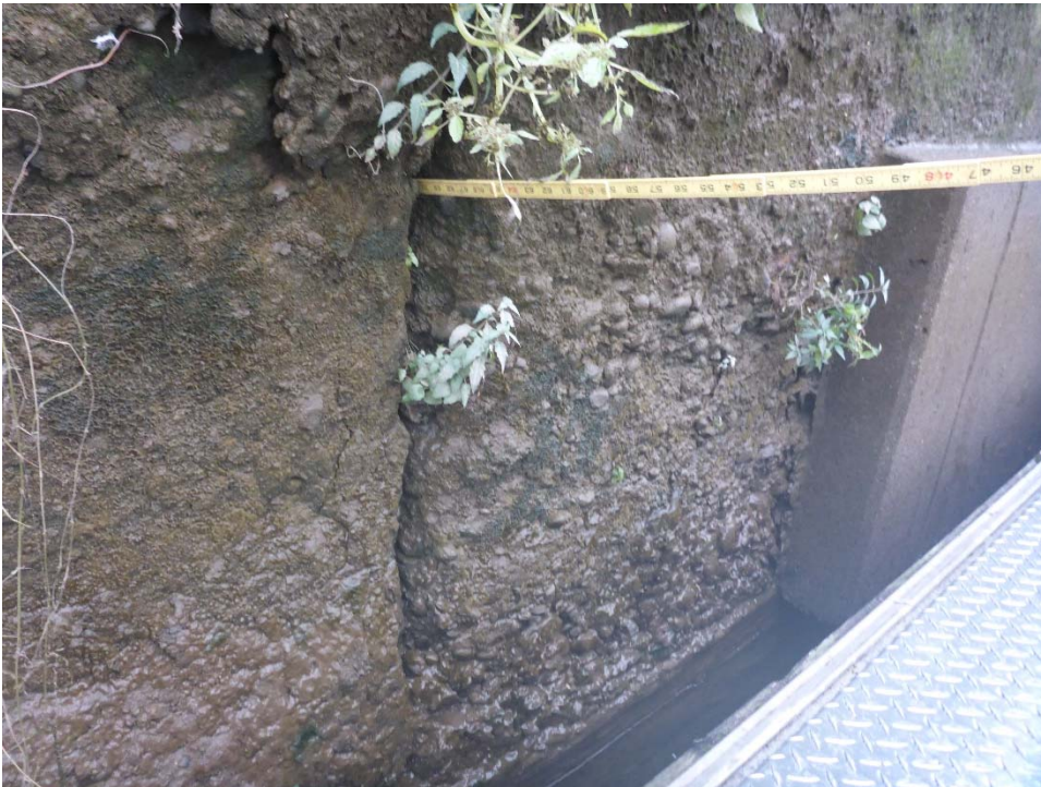
Photo 6: Typical spalling at joint measuring up to 56" H x 4" D approximately 10' west of WD 3.
