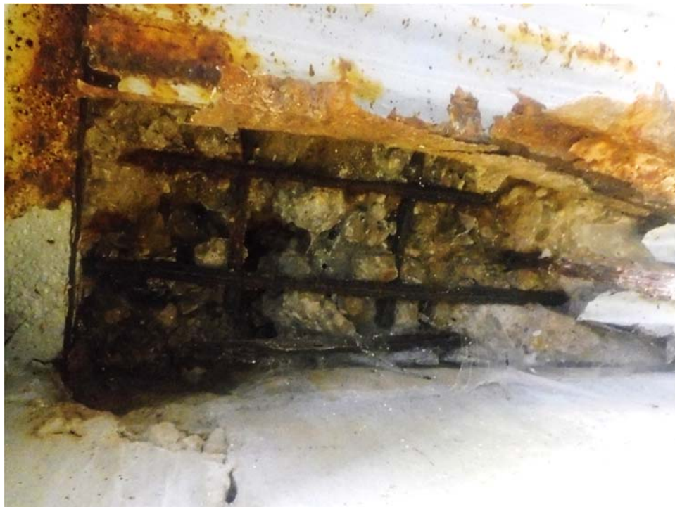
Photo 11: WD 3, east end of Beam 2 from the opening, south side of the beam, looking up. Area of 100% section loss measuring 3' L x 1'W x 9" D to the SIP forms with exposed and deteriorating concrete deck with two layers of exposed reinforcing with up to 100% section loss in the first layer and minor section loss to the second layer. Similar conditions exist on the west end.
