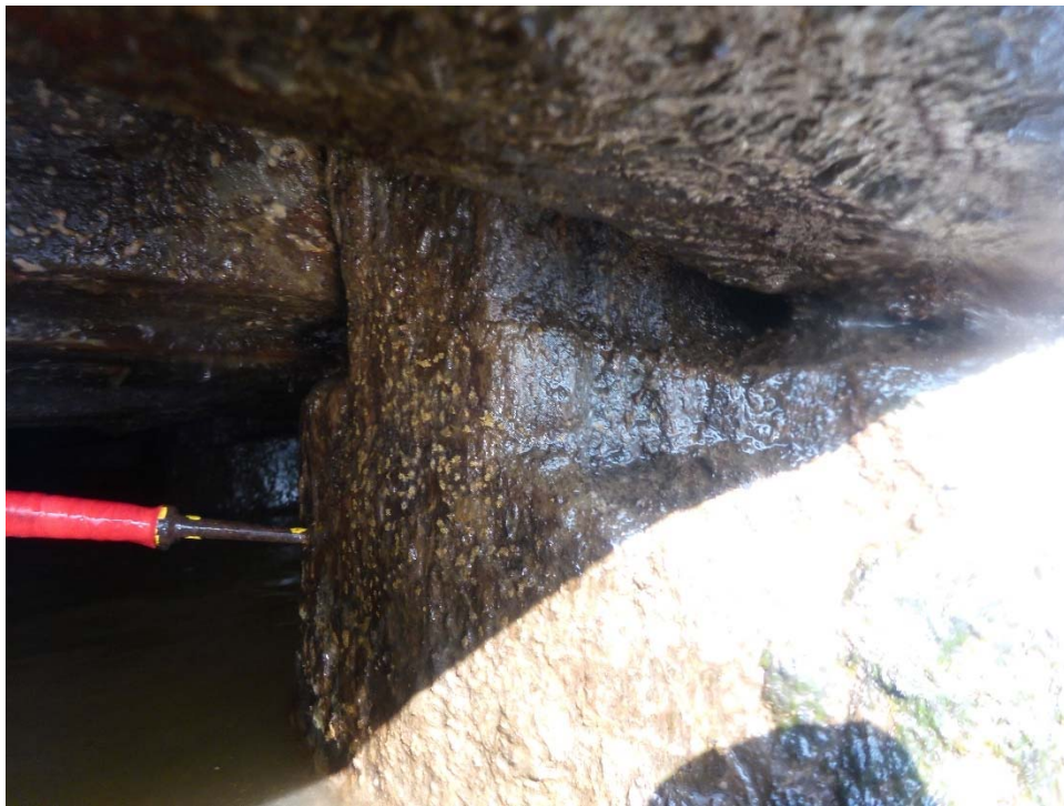
Photo 15: Outshore pile, East face. Typical maximum awl penetration into pile.
