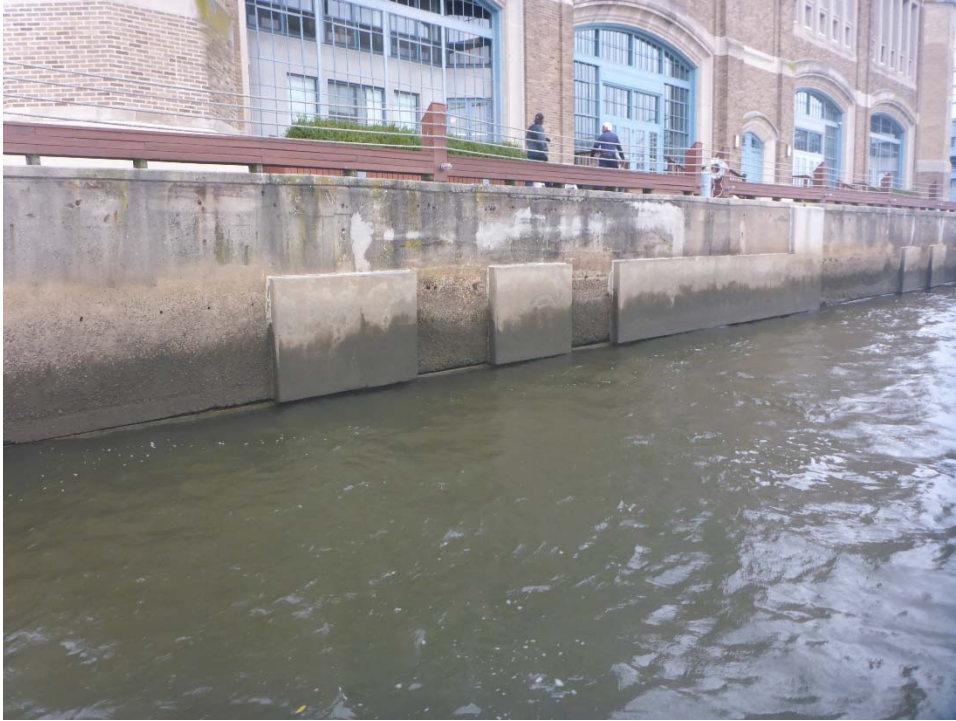
Photo 3: Typical section of east face of pier, looking northwest. The seawall is in generally satisfactory condition with random areas of repairs. Note abrasion in the lower 4' of the seawall, and erosion just above the timber deck.
