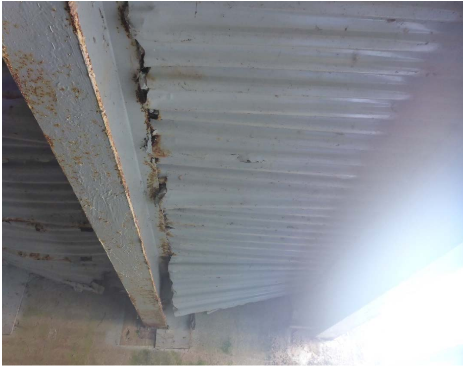
Photo 12: WD 1, Bays 1 & 2 from the opening, looking west. SIP forms have areas of 100% section loss around the perimeters and are bowing downwards.
