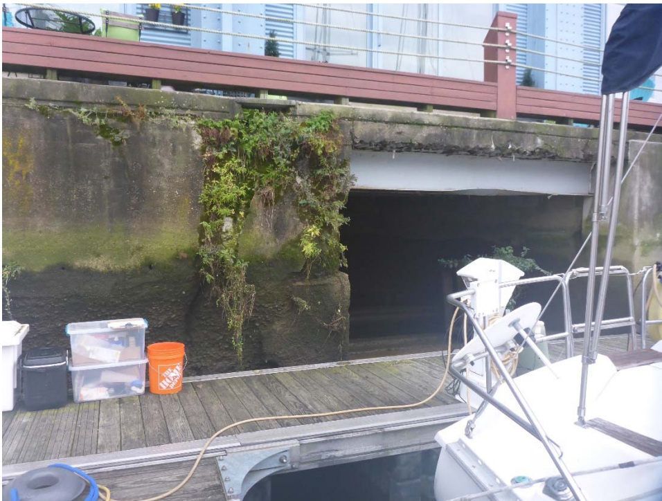
Photo 2: Upper east corner of WD 4, looking south. Full height crack up to 12" deep with significant erosion and spalling at the edges with adjacent hollow area in concrete up to 76" wide. Note heavy vegetation growth. There is ½" to 1" of typical spalling along the top of the wall and moderate abrasion in the lower 4.0'.
