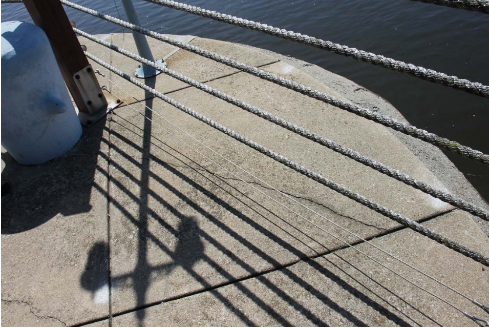
Photo 22: Southeast corner looking east. Localized cracking up to 1/8" W.
