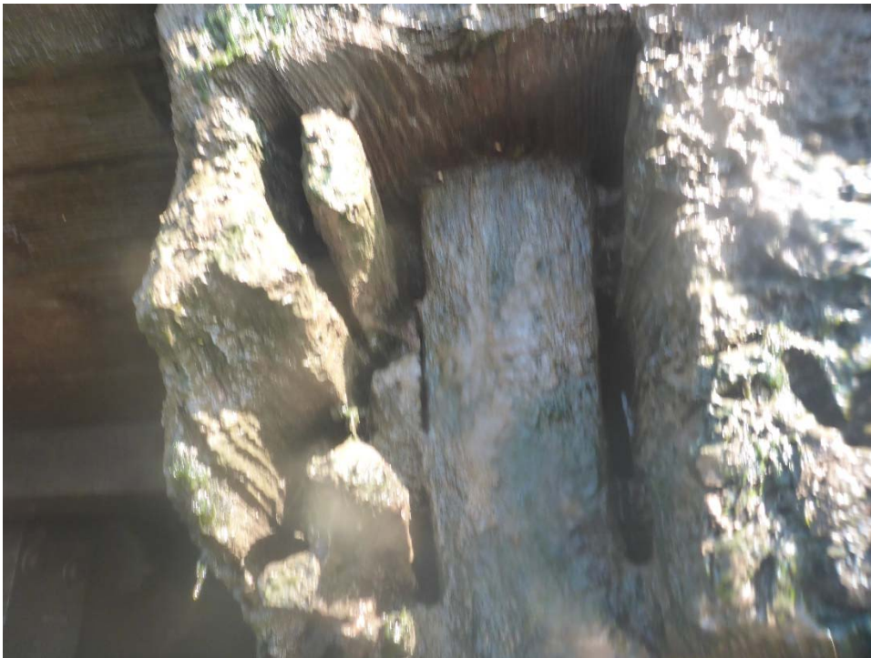
Photo 17: Bent 81S. Timber clamp and cap have deterioration up to 50%
