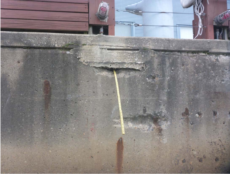
Photo 7: South face. Typical spalling with patch at top of seawall.
